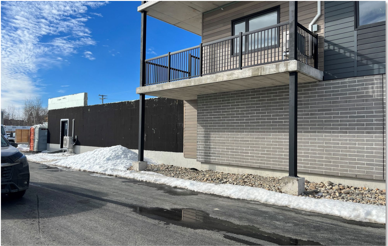
e. Photo 5: exterior view of the main floor and podium (in construction)
